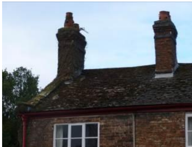
Moss and vegetation to the roof of Big Tree Cottages
