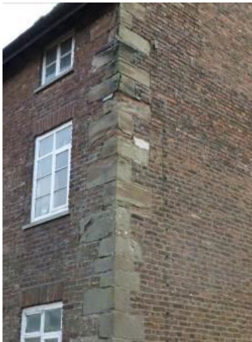
Eroded Quoins to Little Heath Farm House
