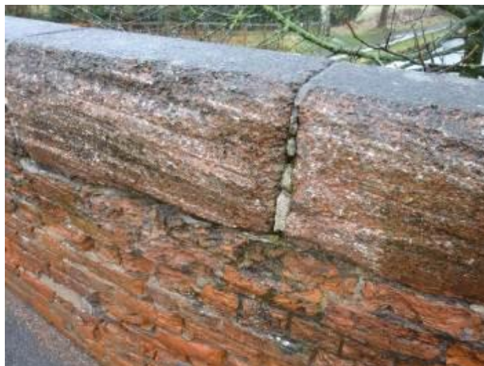
Eroded concrete copings and spalled brickwork below
