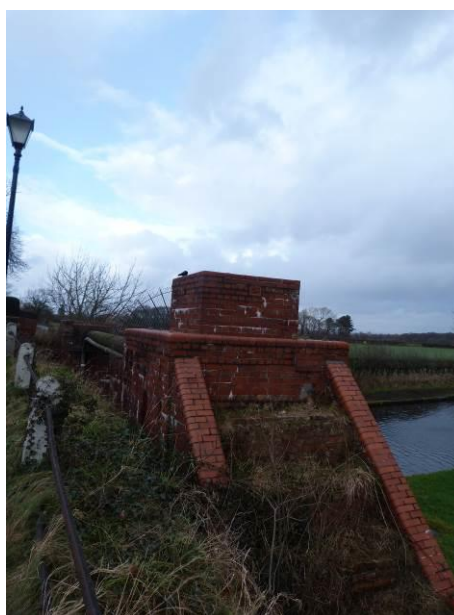
Elevated pipeline by Dunham School Bridge
